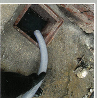
ALWAYS drain the Decarbonizer into a Foul Water drain.
