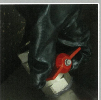
Turn the Red Lever to open the Drain Valve.
